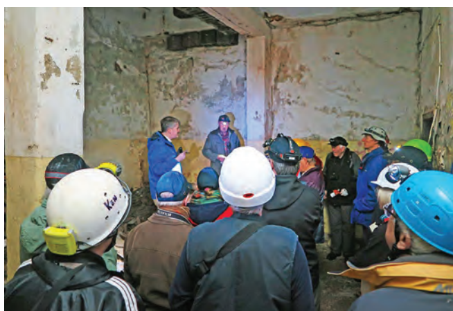
Inside the Koralle bunker, the group gather for a briefing, the general dilapidation evident. Photo Clive Penfold
